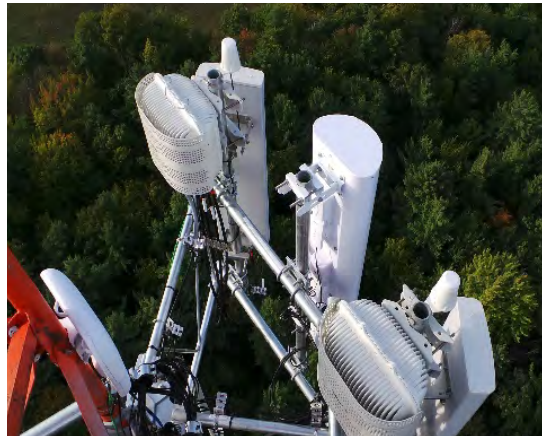
Redzone Wireless 5Gx Network Rural Area Tower Deployment Example
